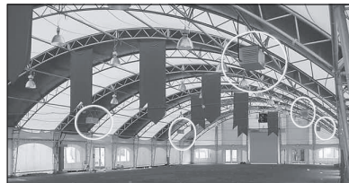
Air being moved in a circular pattern to heat an event tent.
